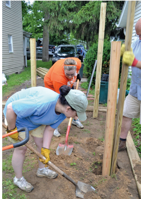
Duane Will and Ryleigh Ewald from Caro, Michigan, and Anissa Mably from Elk River, Minnesota set the initial posts for a handicap ramp during the Fixin' Up The Thumb Servant Event.
